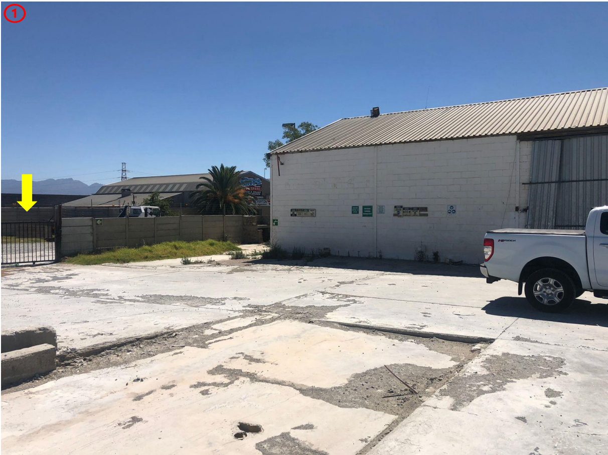
Photograph 1: The existing building, access gate off Carr Street (yellow arrow) and vibcrete boundary wall is visible in this photograph. A ready-mix concrete batching plant previously operated from the site, which is hard serviced for most of its extent. The proponent does not intend to increase the extent of the hard surfaced areas.
