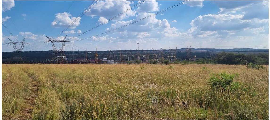
Photo 14: View of Eskom's Carmel Substation taken from the south/south-eastern boundary of the development site, looking south-west towards Carmel Substation.
