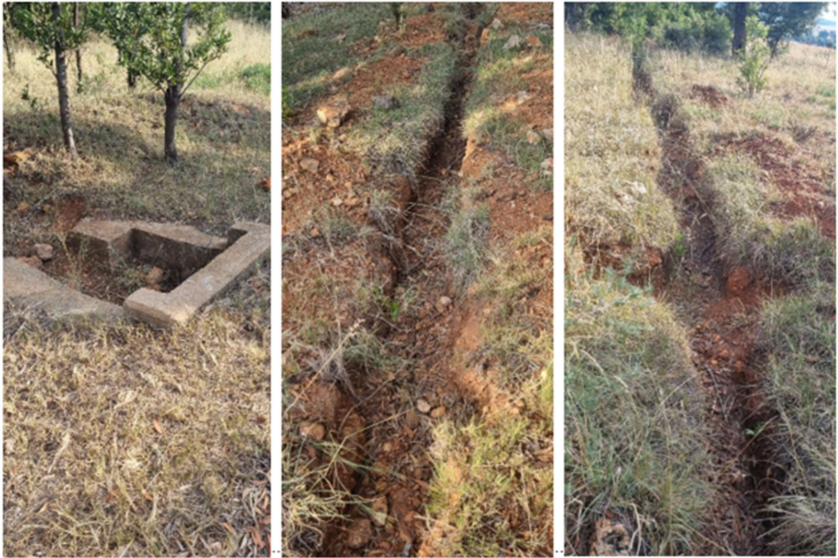
Figure 37: Damaged concrete culvert (left), and old open trenches on the proposed development site.
