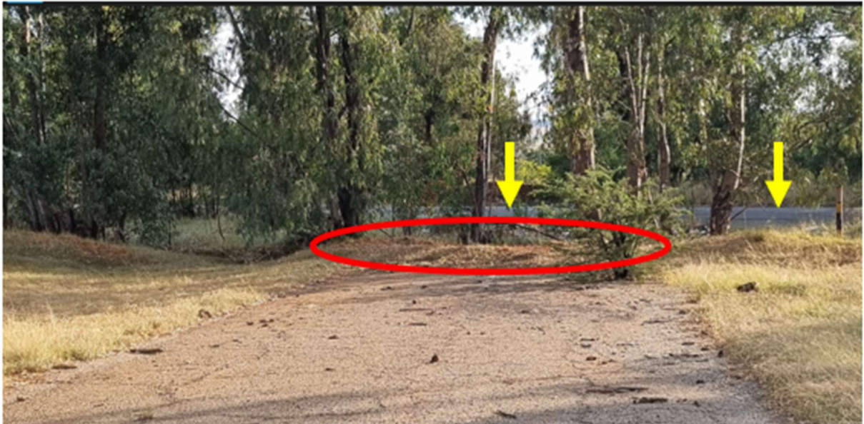
Figure 35: The original intersection of the main access tar road (outlined in red) and the public D92-1020 tar road (indicated with yellow arrows), viewed from within the development site. The intersection will have to be re-established/repaired.
