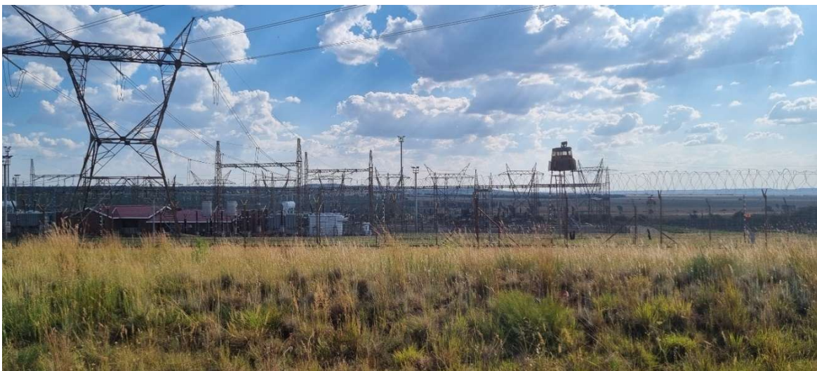
Figure 32: View of Carmel MTS from the east/south-eastern corner of the substation. Infrastructure lies immediately to the south of the proposed development site.
