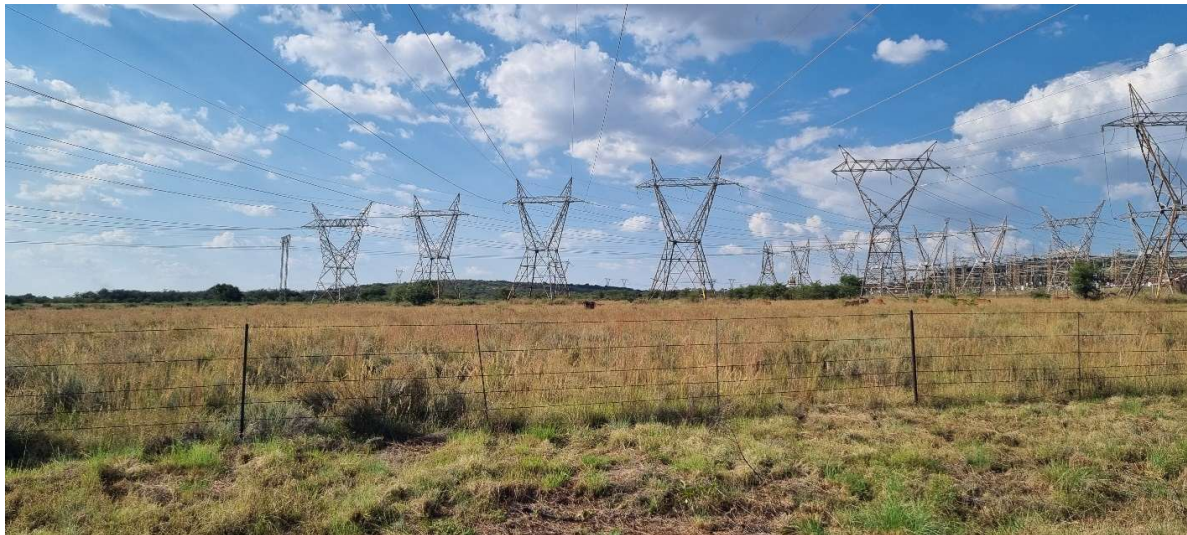
Figure 30: Eskom's HV OPL steel lattice pylons entering Carmel MTS from the west. The proposed development site is on the left-hand side background of the image.
