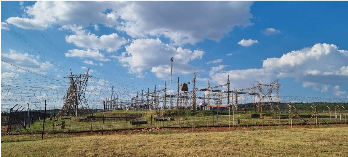
Figure 31: Eskom's HV OPLs at the south-western boundary of Carmel MTS.
